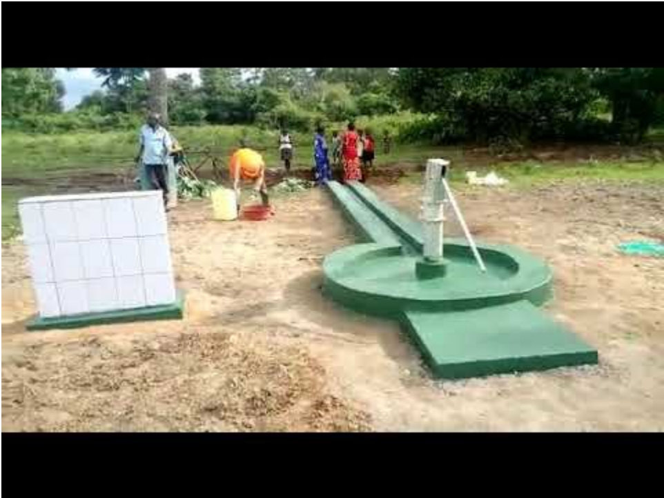
Community Borehole Infrastructure/ Unit
